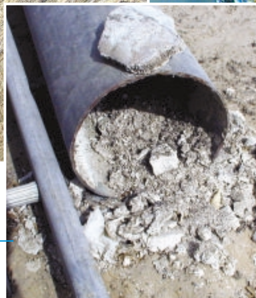
Deposits of CaSO 4 in a sludge pipe
